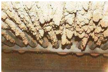
Heating surface before cleaning
